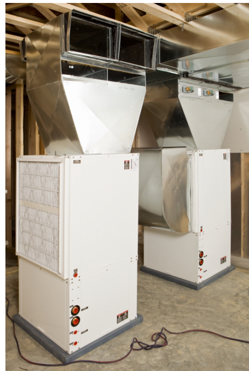
Geothermal HVAC units can heat and cool the home very efficiently
